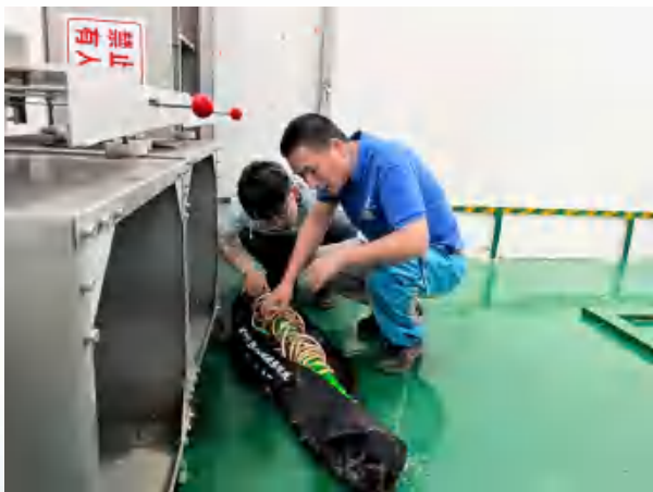
Shanghai Haichang Ocean Park Conducted 10kV Substation Inspection 上海海昌海洋公園開展10kV變電所檢查
